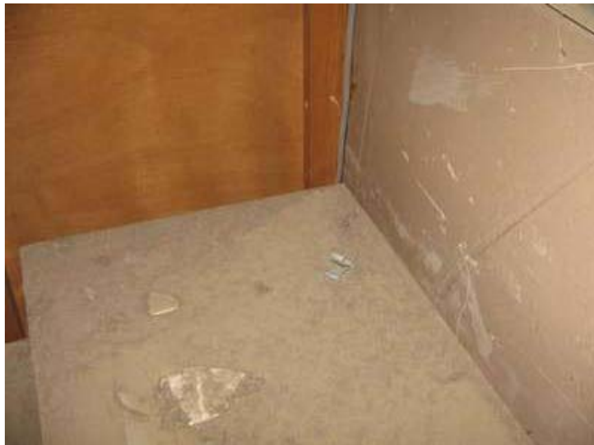
Unsealed, damaged AIB and debris within a heating cabinet
